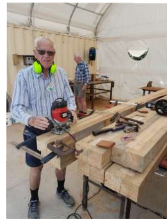
Shedder Michael Galloway working on the pergola uprights which will have the six panels inset into them.
